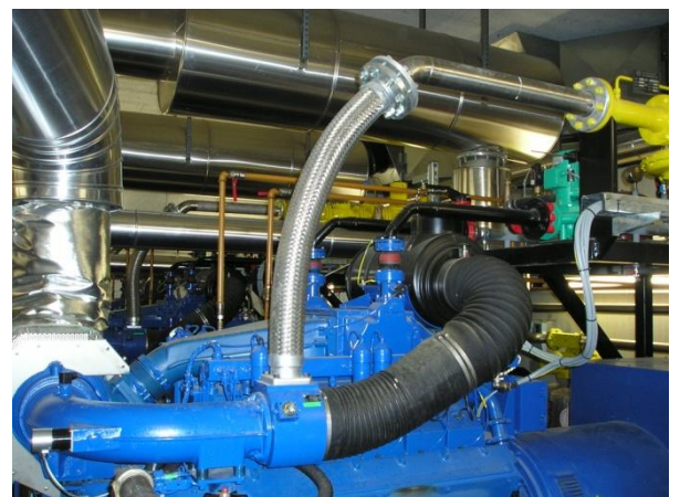
co-generation unit 1.500 kW el with transformator
